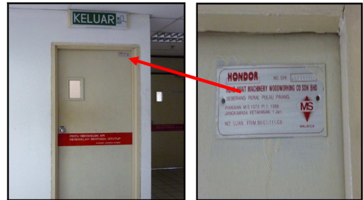
The fire door and the certification of the fire door
